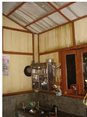
Badly leaking kitchen roof in our houses – Sept 2010
