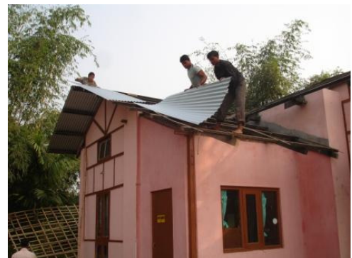
Getting a new roof – Jan 2011; thanks to Caring Friends, no more getting up in the middle of a rainy night to catch water in pots and pans!
